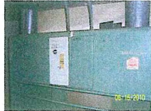
Figure 5: Furnace on lower level
