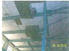
Figure 6: Ductwork for gym
